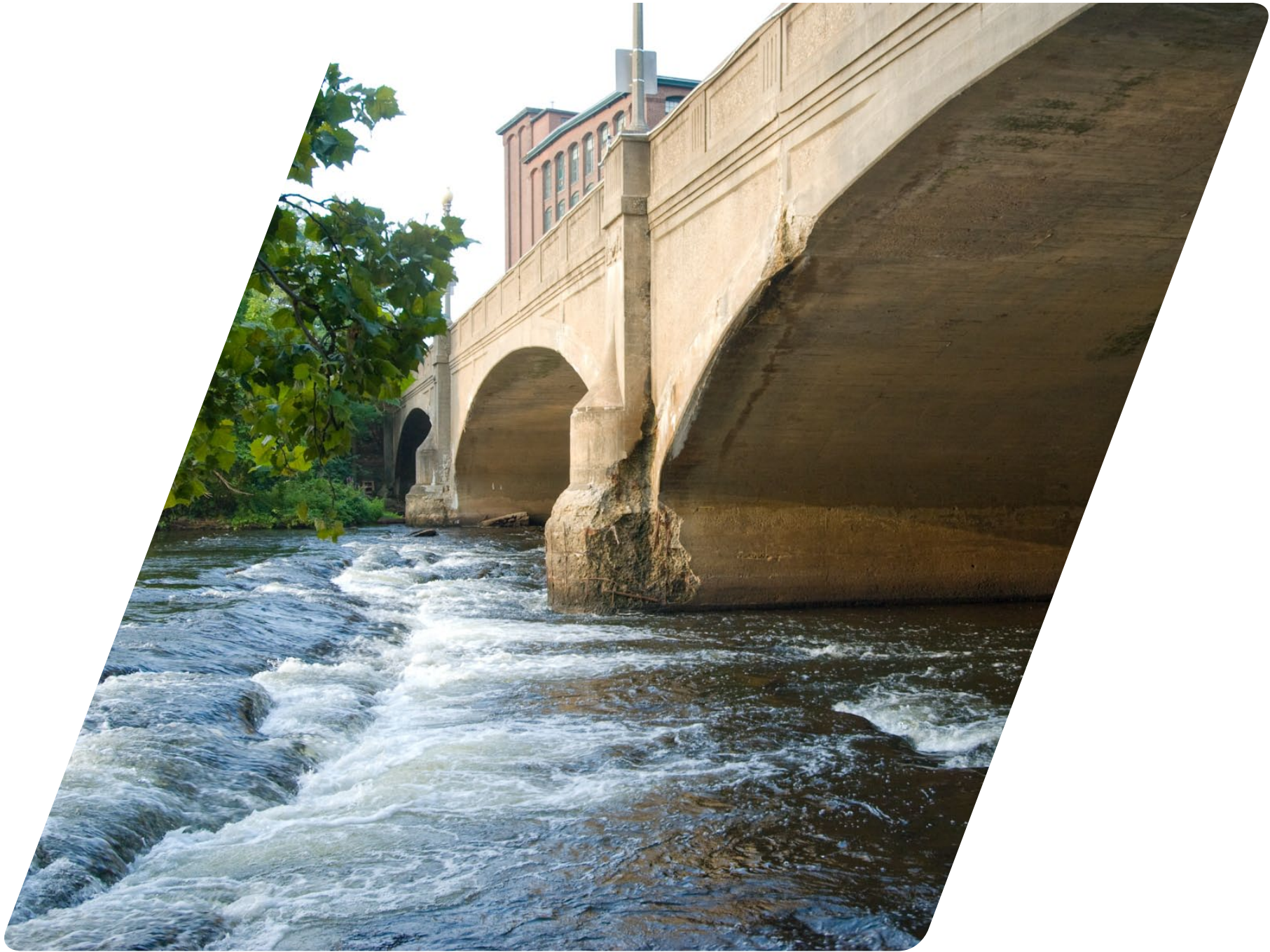
Water damaged abutments of Davitt Memorial Bridge
