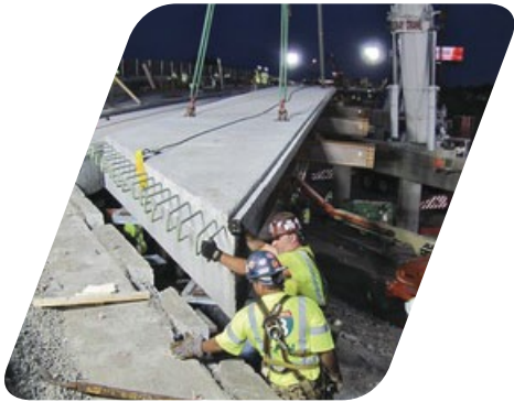
Innovation – Award-winning Fast 14 rapid bridge replacement saved millions of dollars and valuable time on I-93 by using innovative techniques – Medford
