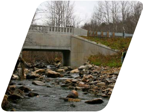
Sustainability – Award-winning project that replaced a bridge and improved the environment at the same time – Becket
